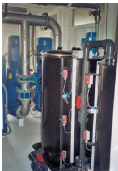
Aluminium sulphate dosing equipment
