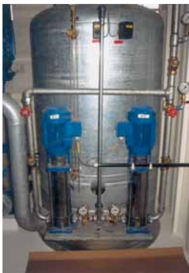
Booster pumps for water/ chlorine dosing
