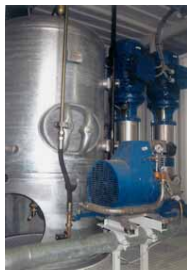
Pressure tank and compressor
