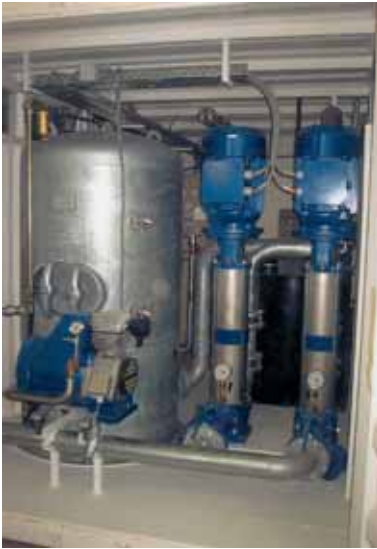
High lift pumps 50 m 3 /h 80 m
