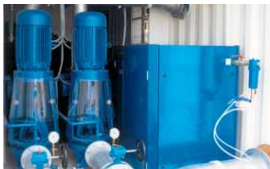
Low lift pumps and blower
