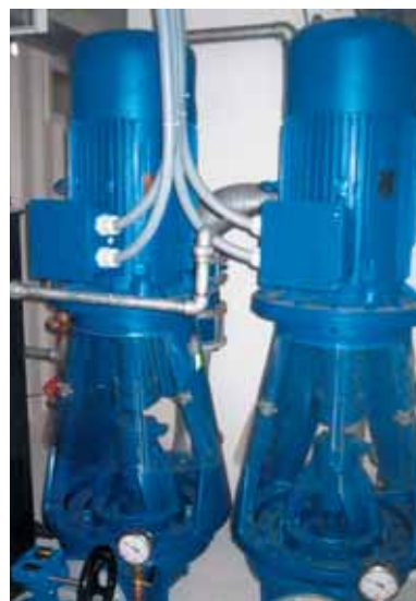
High lift pumps 240 m 3 /h 50m
