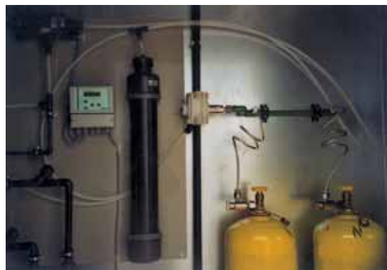
Chlorine gas disinfection
