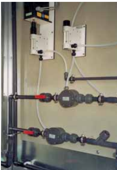
Chlorine gas disinfection
