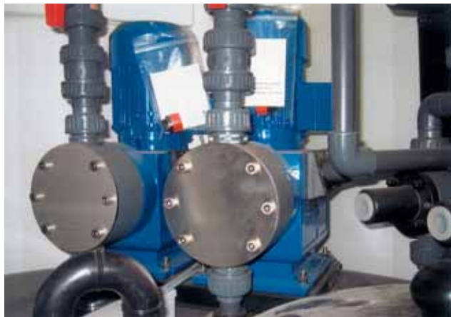
Aluminium sulphate dosing pumps
