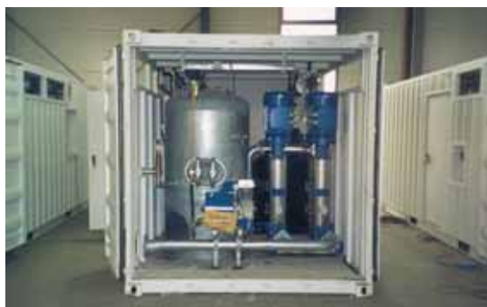
High lift pumps, pressure tank and compressor
