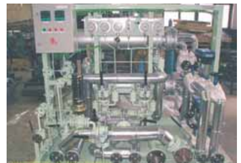
Fuel oil conditioning unit for boiler's burner
