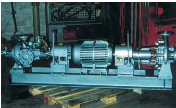
Electrically driven cooling water and ballast pumps with clutches
